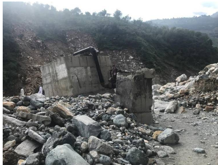
Damaged Drainage Valve for Siphon
