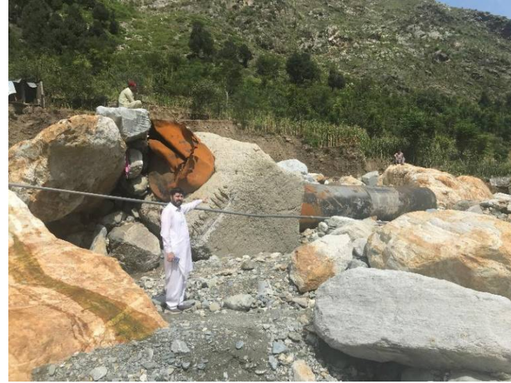
Washed away piece of Siphon
