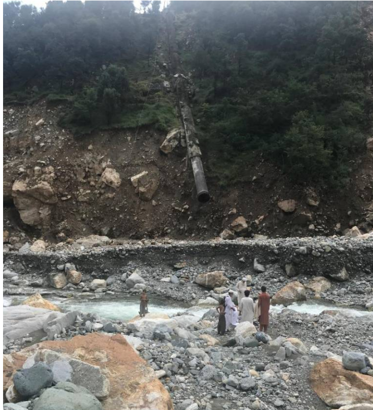
Damaged portion of Siphon
